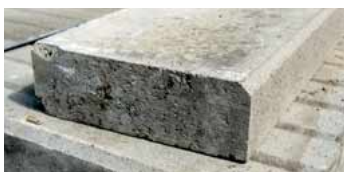
Old concrete, concrete
