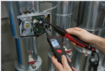
Voltage test AC
